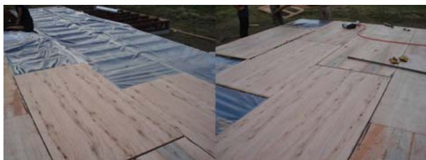
Figura 5. Colocación de tableros fenólicos de 10 mm. Figure 5. Positioning of phenolic boards with 10 mm.
