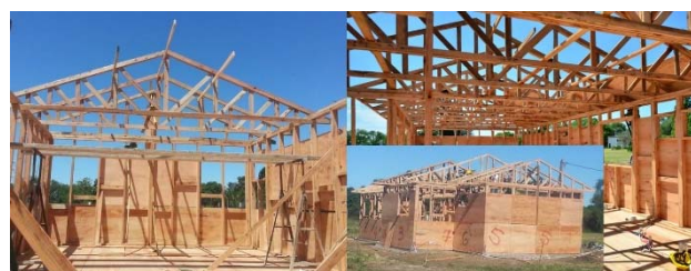
Figura 8. Colocación de tímpanos, cabriadas y tableros fenólicos faltantes. Figure 8. Positioning of trusses and phenolic boards.
